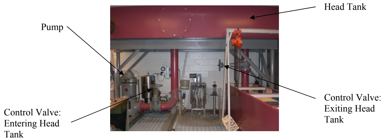
FIG. 6. Head Tank and Control Valves
